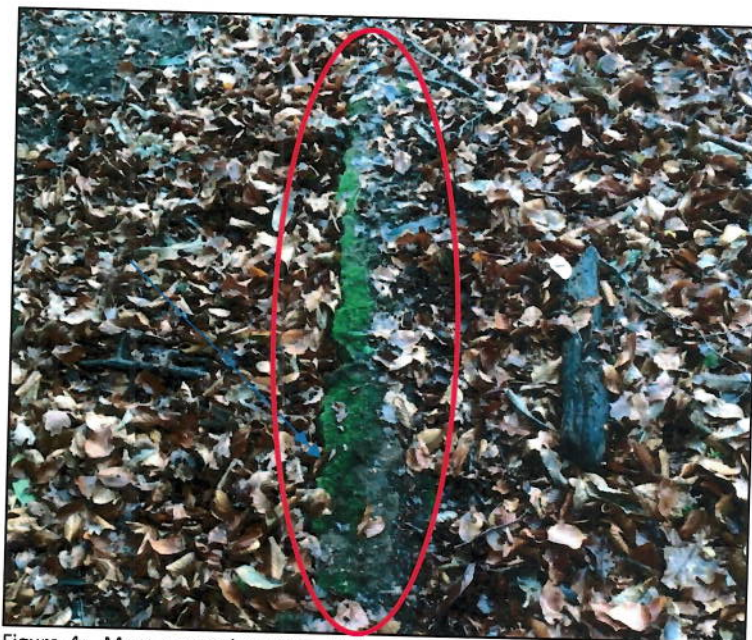
Figure 4: Moss-covered section of the western garden boundary wall (ringed in red) seen on the second site visit and highlighted in Figure 3 above
